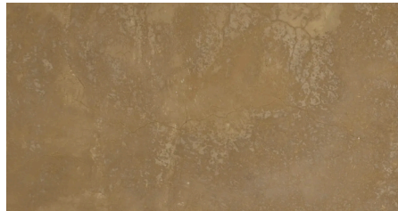
Copper Gutters & RWLs
