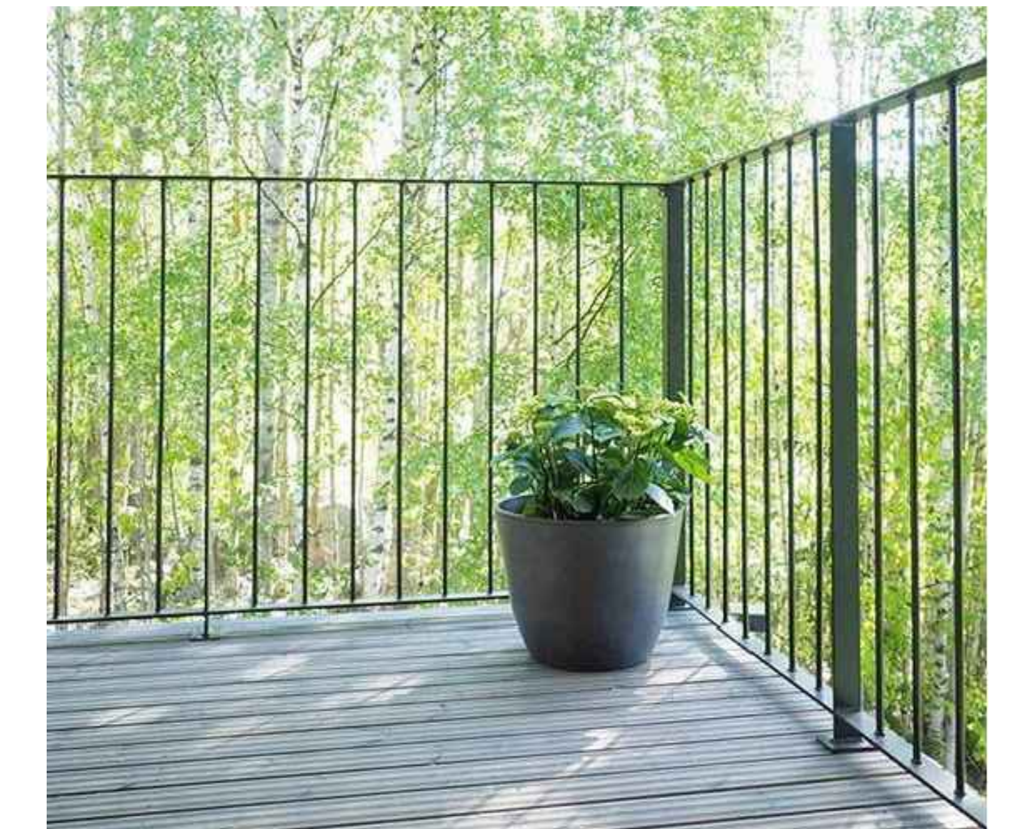
GUARDRAILS MATERIALS: STEEL; PAINTED
